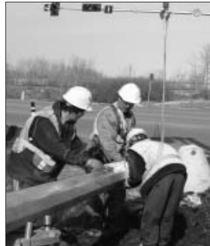
Workers re-install traffic lights on Highway 15 south of the Scotford Upgrader. Installation of the lights will be completed in advance of the Shell Scotford Upgrader spring maintenance turnaround.
